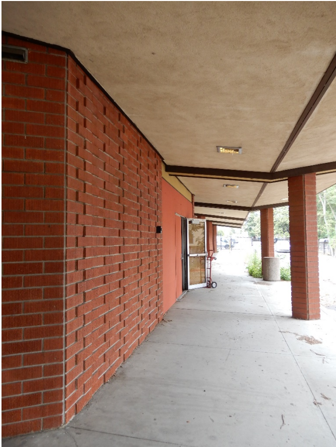
Figure 4. South façade, view east showing façade, column, and eave detail (ARG, July 2021)
