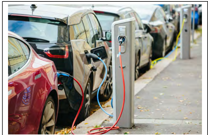
Curbside Electric Vehicle Charging
