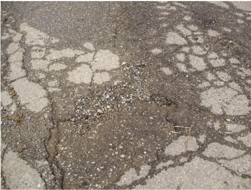
Photos C, D and E showing totally non-functional, non-maintained by County, inadequate drainage system in front of our property
