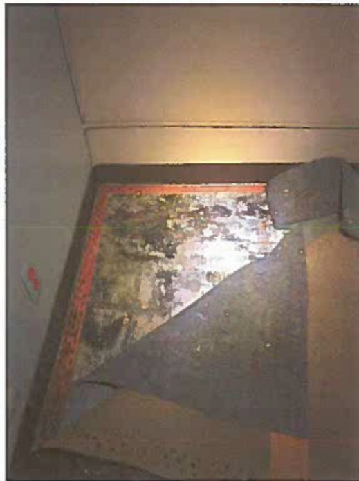
Photo 16 – No vinyl floor tile in Basement
