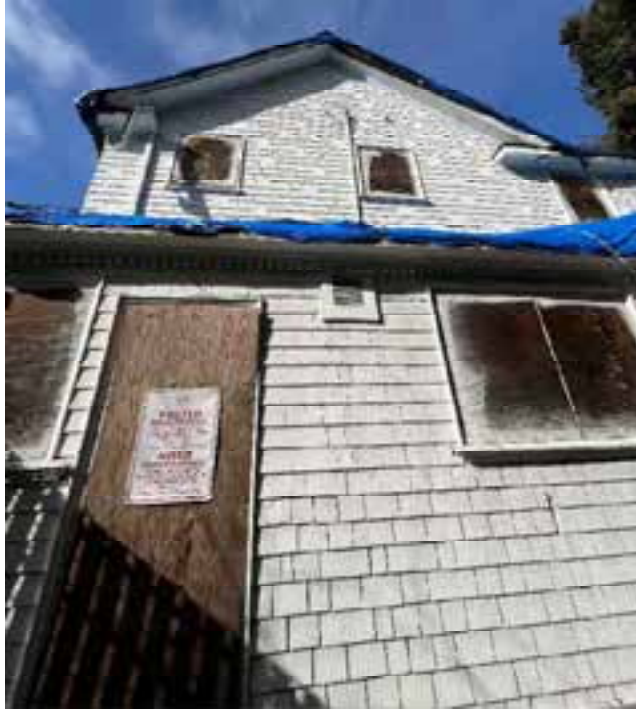
Figure 6. East elevation, center bay.
